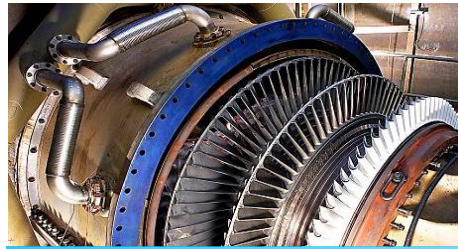
Steam and gas turbines
